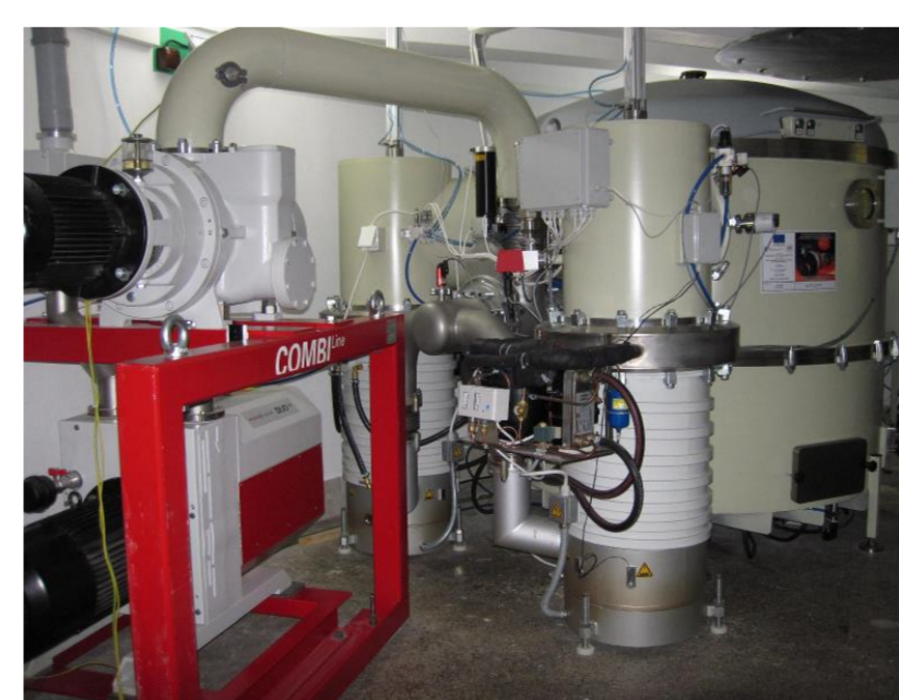
Mirror coating facility
